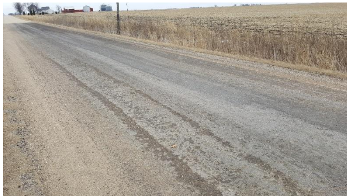
MC-70 Road Oil was applied over the crushed stone road approximately 8 months prior to the picture for dust suppression. Proper maintenance by the owner will result in a long lasting product.
