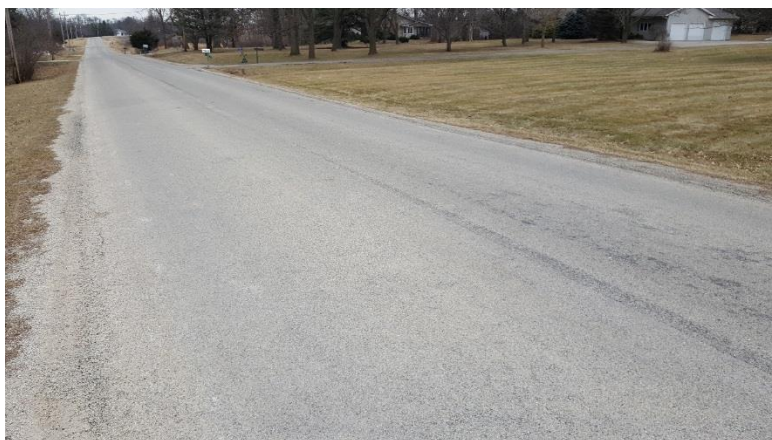
MC-3000 Seal Coat was applied over the crushed stone road approximately 2 years prior to the picture for dust suppression. Weather and traffic have turned the Seal Coat to a grey color with minimal dust. Proper maintenance by the owner will result in a long lasting product.
